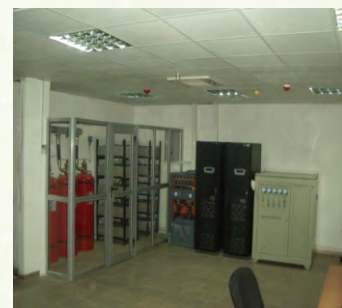
MDAs Server, UPS & Stabilizer Room
